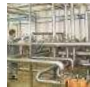
Company owned test center for new developments and product control
