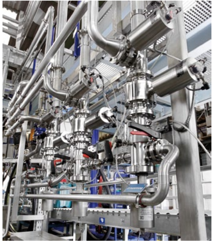
KIESELMANN pigging system in a production plant
